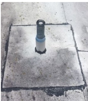
Typical permanent roof anchor point
