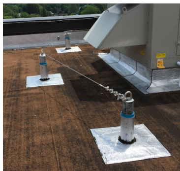
Typical permanent combination anchor point and lifeline
